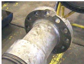
Figure 1. Damaged coupling due to an explosion event
