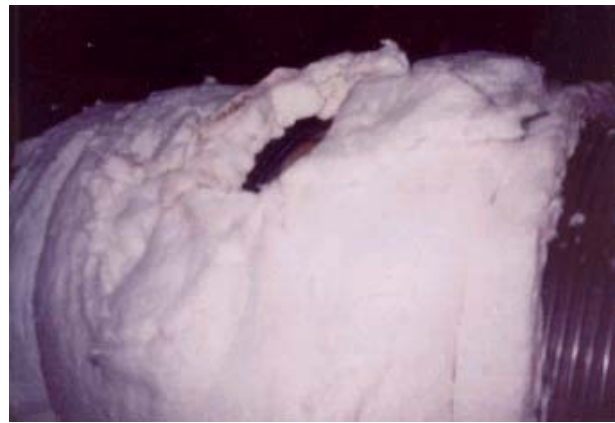
Figure 6. Utilization of locally hot spotting on bent rotor with dry insulation.
