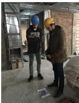
Figure 2. Scanning QR code to link an upper floor unit to the corresponding elements of the model unit
