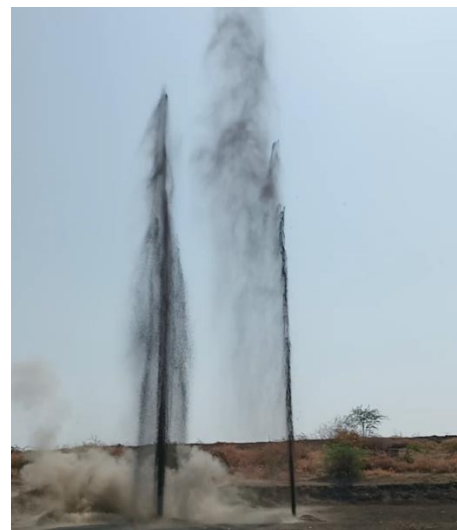
Figure 6. Water upliftment due to explosion
