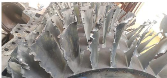
Figure 1. Damaged turbine in the Kirkuk gas power plant (severe destruction of blades)
