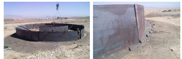
Figure 2. Circumferential sheets installation process in the body of tank and generation of different imperfections
