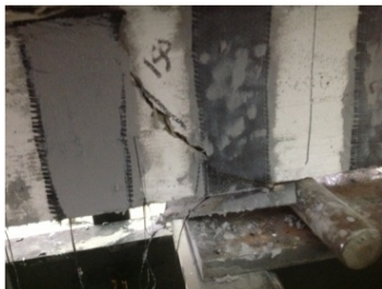
Figure 4. Cracking and failure pattern of beam B2.5-U-S
