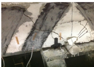
Figure 5. Cracking and failure pattern of beam B2.5-L-S
