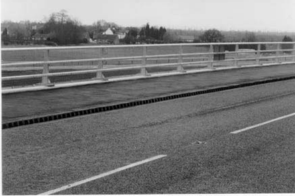
Figure 3. The finished view of the CIS Bridgeflow II drainage channel units (after road asphaltting).
