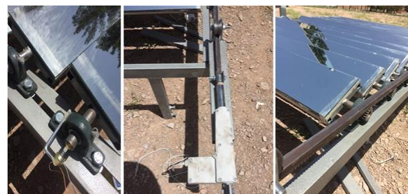
Figure 7. The developed solar tracking system
