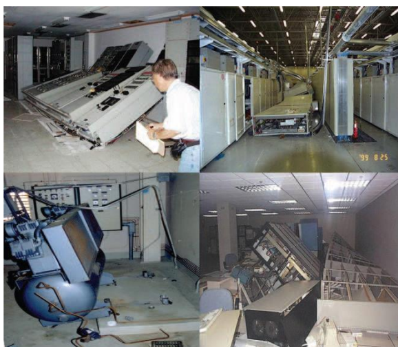
Figure 2. Earthquake damage of NSCs [5]
