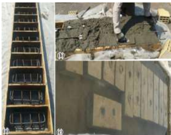
Figure 3. Construction and curing of the beams a: Formwork and reinforcement b: Concreting c: Curing
