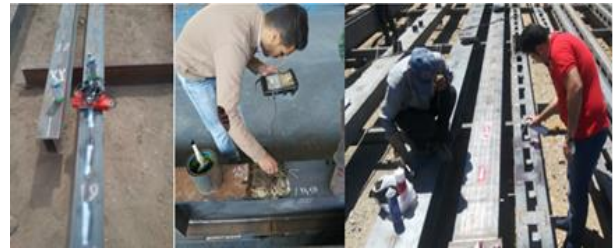
Figure 4. Welding defects tested by different methods (left to right: MT, UT and Penetration test)
