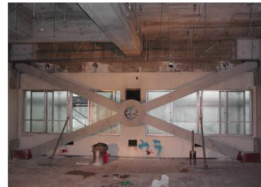
Figure 3. The X-shape concrete brace placed in the existing frame (Enough openings still exist.)
