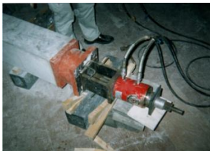
Figure 1. Introduction of prestressing force to the lower part of a diagonal member
