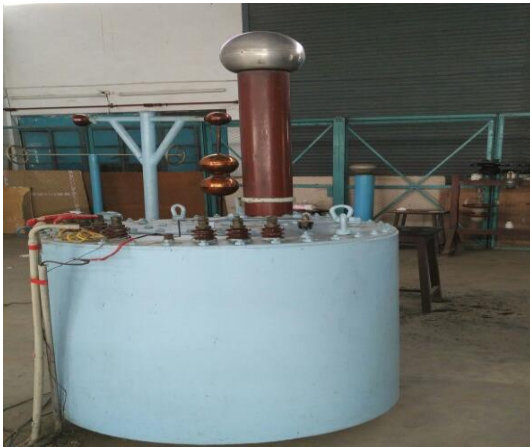
Figure 2. Transformer of 391V/150 KV, I-phase 30 KVA
