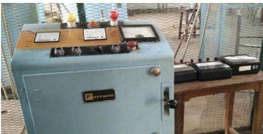
Figure 3. Voltage regulator at primary side of transformer
