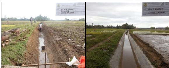
Figure 1. Construction of concrete lining on tertiary irrigation channels in the Batang Anai Irrigation Project in West Sumatra Province
