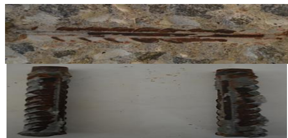
Figure 14. Condition of concrete and coated rebar at the end of the test
