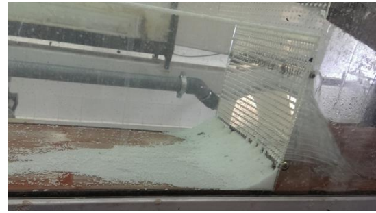
Figure 10. Accumulation of sediments upstream obstacle
